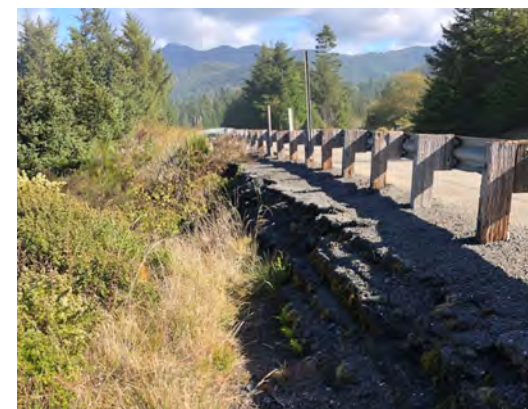
Multiple layers of asphalt pavement on US 101 southbound shoulder indicating ongoing displacements.
