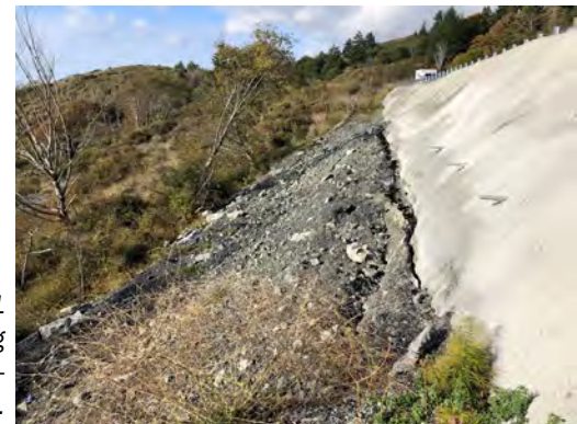
Localized failure of the slope below US 101 southbound. The failure caused damage to the existing soil nail stabilization including an approximate one-foot gap at the bottom of the shotcrete facing.
