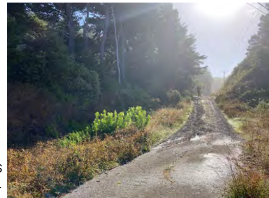
Vertical offset and pavement damage on Old US 101 along the southern margin of the slide.
