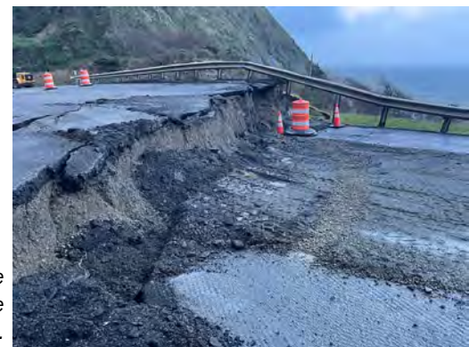
A 2023 slide near the Arizona State Recreational site along U.S. 101 dropped the roadway by as much as 12 feet in some places.
